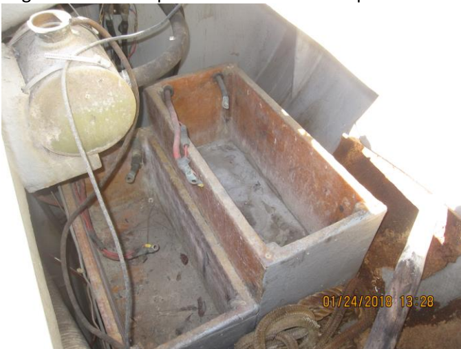
Battery boxes and old battery cables
