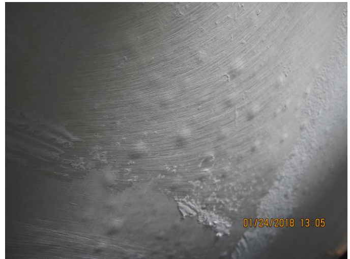
Dense very small diameter (3/8-inch) osmotic blisters, sporadically throughout wetted surface hull
