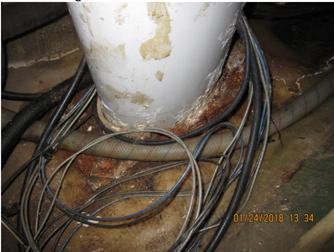
Corrosion at base of main mast
