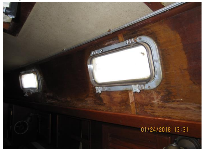
Water damaged wood around all portlights
