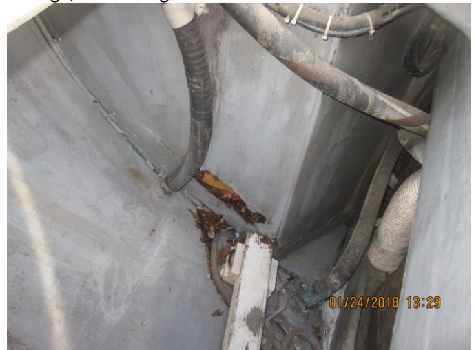
Water damaged minor bulkhead at forward end of port cockpit locker
