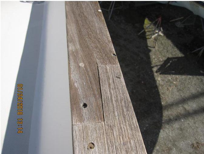
Many exposed toe rail plank fasteners exposed
