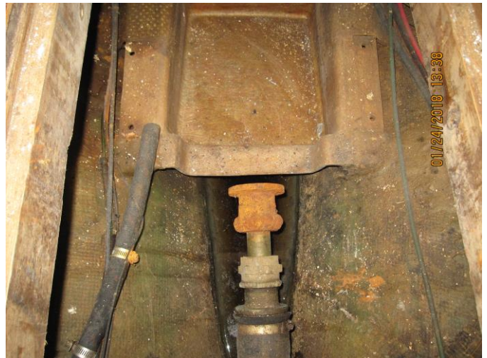
Walter vee-drive missing
